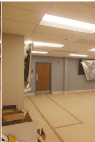
Spaces in Rhodehouse Science Building are being renovated for the physician assistant and speech-language pathology programs. Students will begin using those spaces in July.
