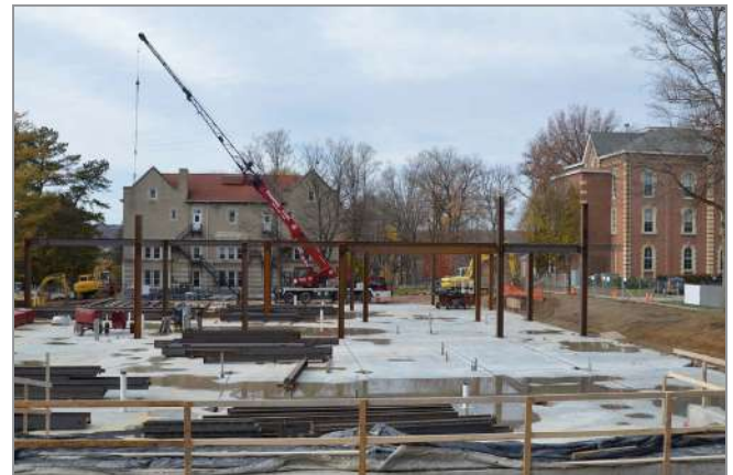
The James Pedas Communication Center is taking shape! As of Nov. 9, the cement slab has been poured and the steel beams are being set.
